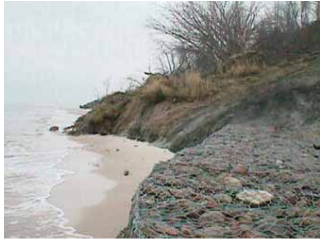
Fig. 6. Seawall built in 1994 for protection of the cliff, partly destroyed by landslide in January 1999 (Photo. by Sz. Uścińowicz)
