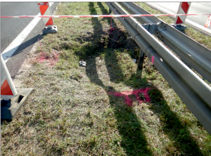
Ryc. 9. Lej zapadliskowy w pasie zieleni DK 94. Fot. J. Kos Fig. 9. A sinkhole in the green belt of DK 94 road. Photo by J. Kos
